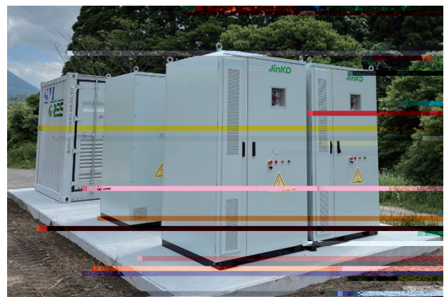
Fig. 2 Jinko ESS 215kWh DC Blocks
